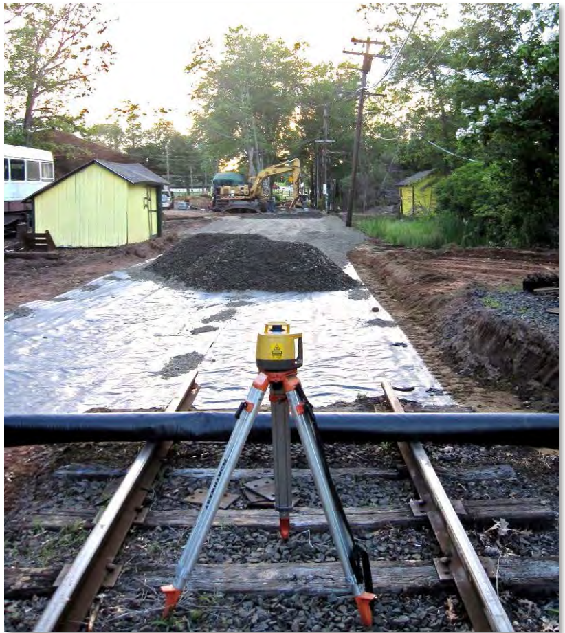
Looking Westbound during the complete replacement of 210 feet of mainline track at the Members Crossing.
