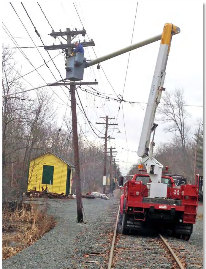
John Arel using the Museum's bucket truck while performing repairs on the Museum's highline.
